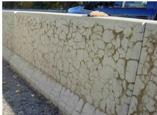
Cracks in a median highway barrier affected by ASR [3]
