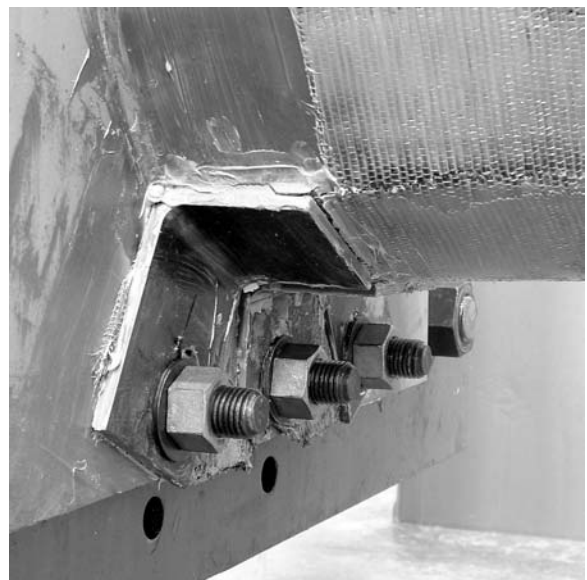
Figure 16 Rupture of the CFRP sheets on the tension side of the base
