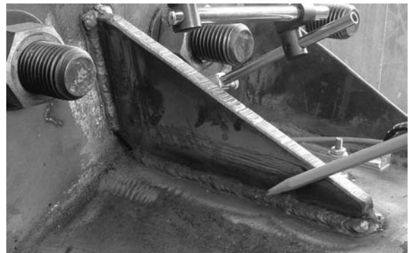
Figure 12 Gusset plate welded from the corner of two flats on the monopole shaft to the base plate
