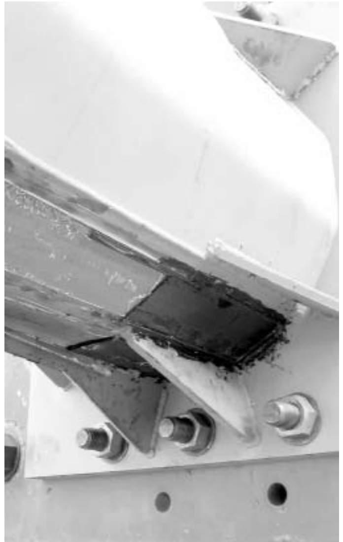
Figure 8. Rupture of CFRP strips at end of gusset plates for monopole (MAB-H).
