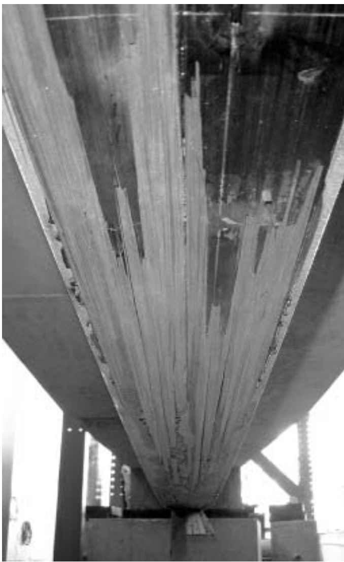
Figure 14. Soffit of girder (CGAB-I) showing interlaminar shear failure of CFRP strip away from midspan.
