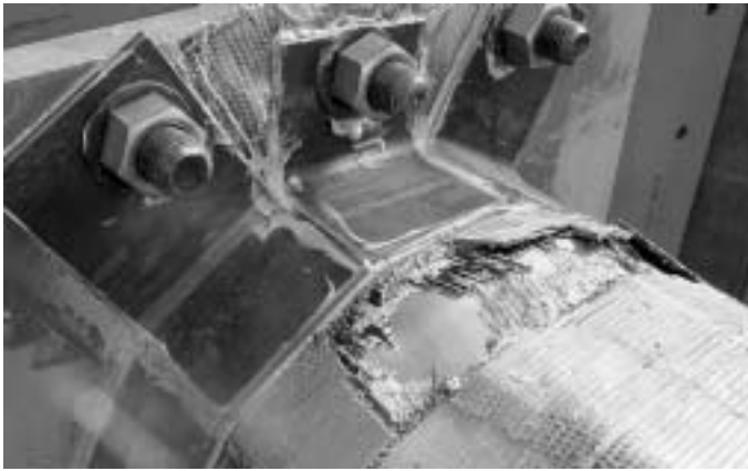
Figure 6. Detail of local buckling at base showing anchorage angles for sheets.
